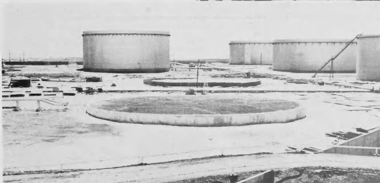
LOOKING LIKE a splattered lime in the aerial view above is an old spheroid, one of the many of this design currently being dismantled and replaced by the standard, familiar tank. Foundations for the replacement storage tanks take shape, above.
